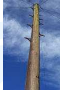
Step bolts on pole
